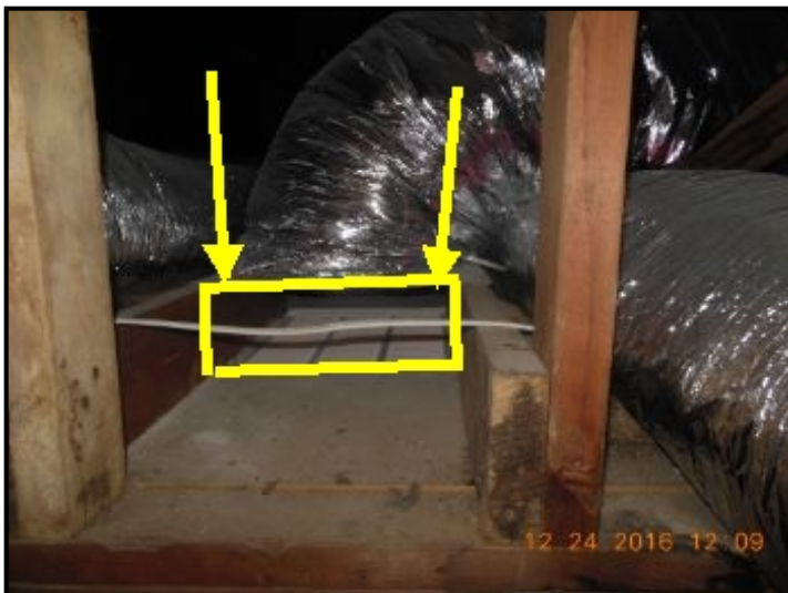
Wide open gaps noted at return duct flange and ceiling register
