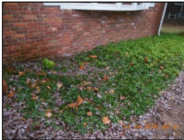
Grounds are settled significantly at front side of home
