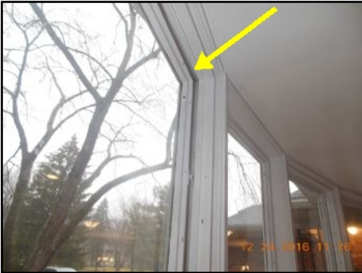
Casement window is stuck at top side
