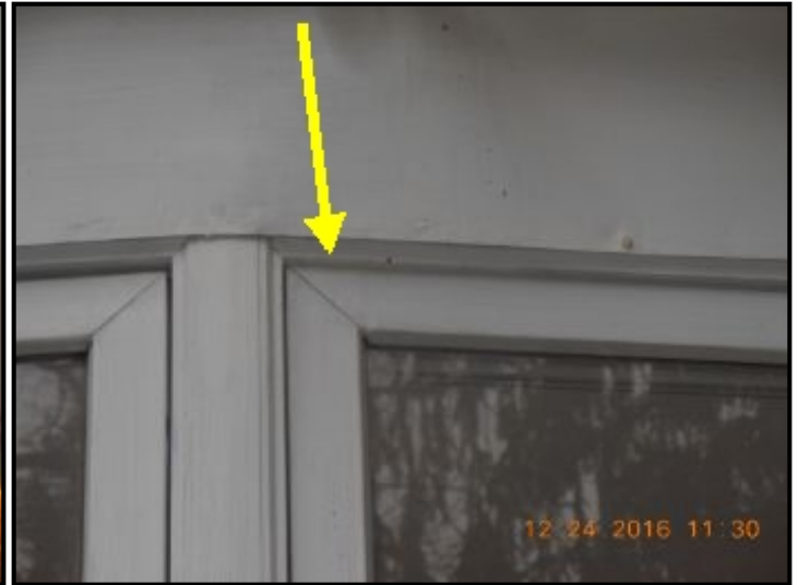
Casement window is stuck at top side
