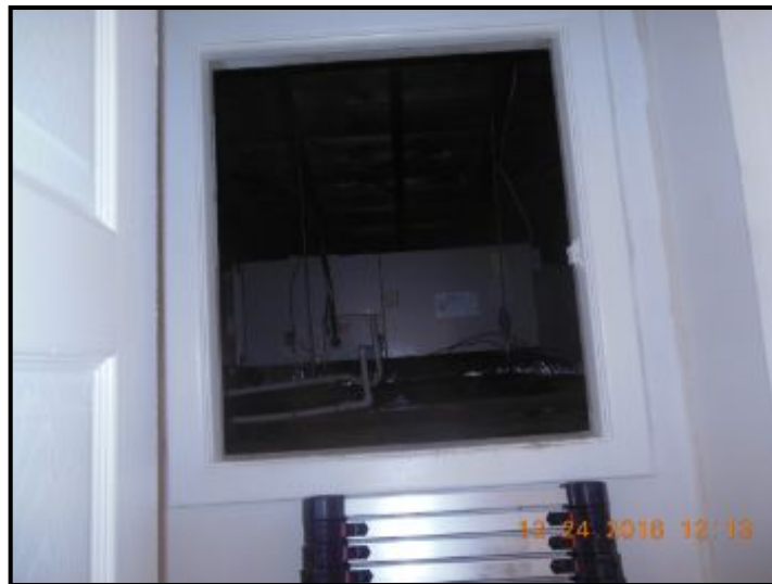
Missing door noted at attic access opening
