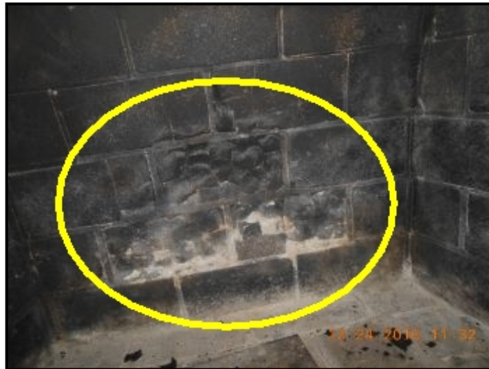
Back wall in fireplace is significantly damaged
