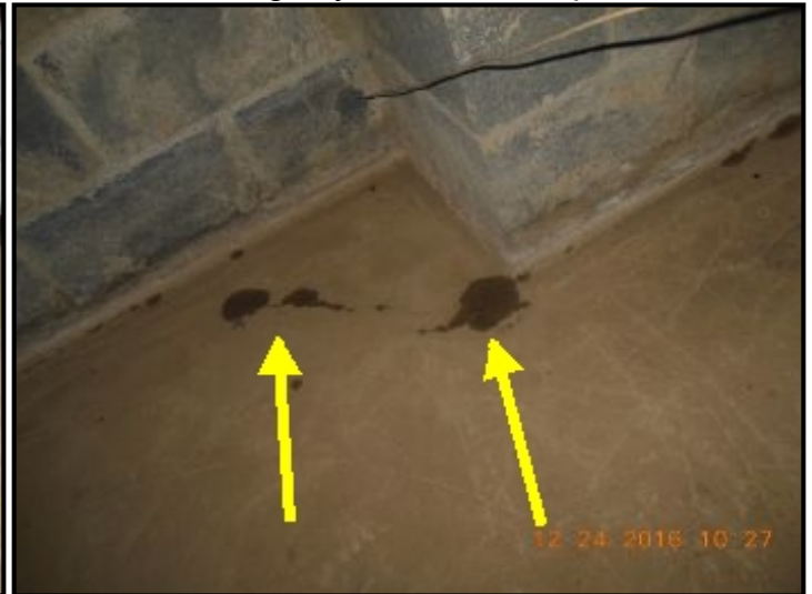
Wet spots on floor next to fireplace indicates water control in crawlspace is inadequate
