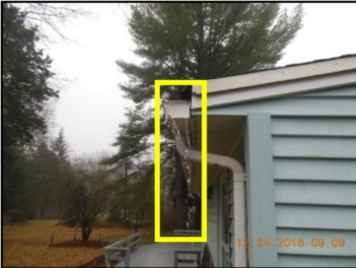
Gutters are overflowing from heavy leaf buildup in gutters
