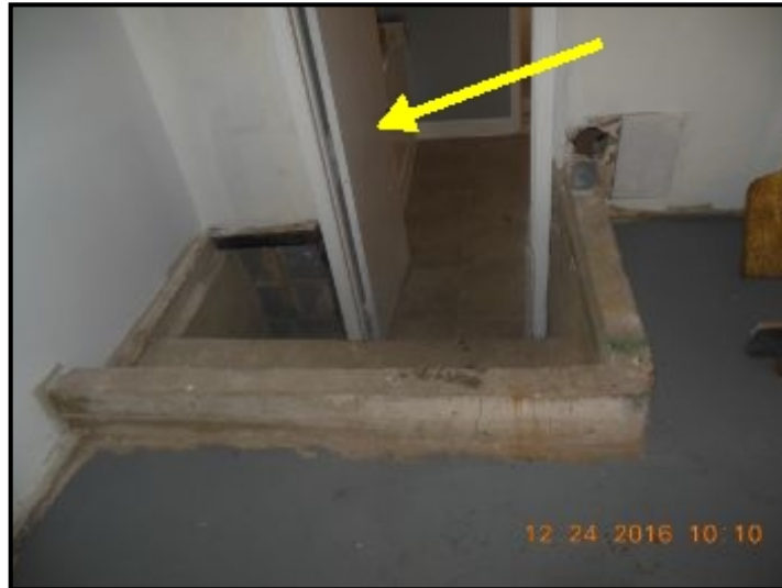
Fire door does not close automatically when released
