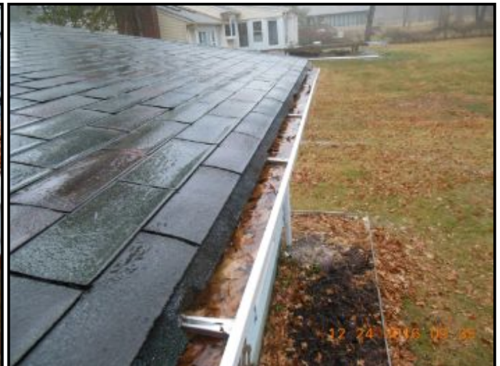
Gutters are full of leaves and overflowing
