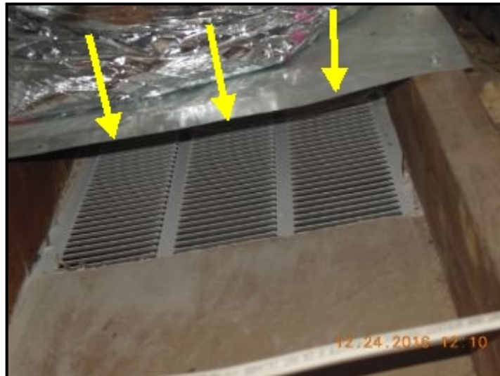
Another angle showing wide open holes between return duct flange and ceiling
