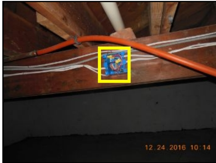
Open junction box noted in crawlspace
