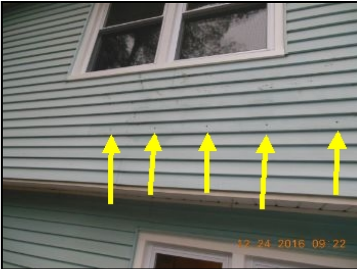
Open holes were noted in vinyl siding from removed deck awning cover
