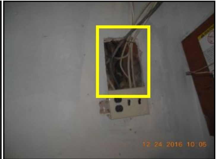
Open hole noted on firewall in garage
