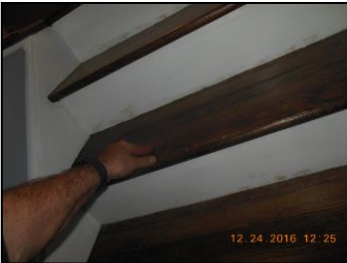
Several loose step planks noted at stairs
