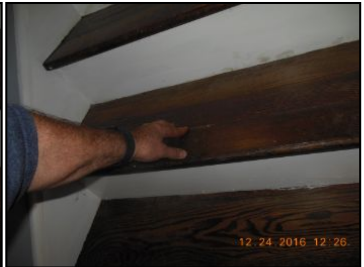
Several loose step planks noted at stairs
