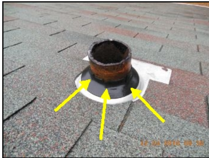
Cracked neoprene collar noted around plumbing vent pipe
