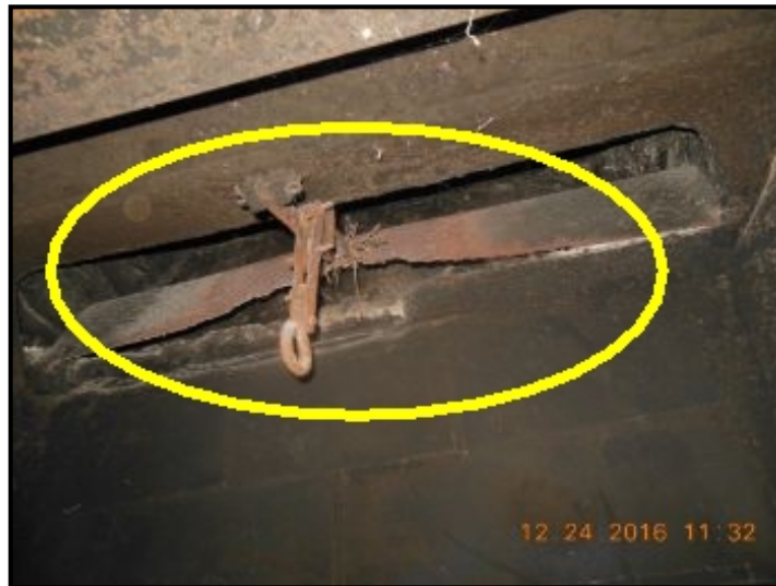
Damper is rusted out with wide open hole
