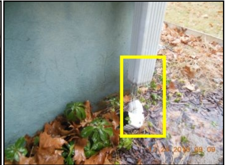
Downspout is draining next to foundation walls
