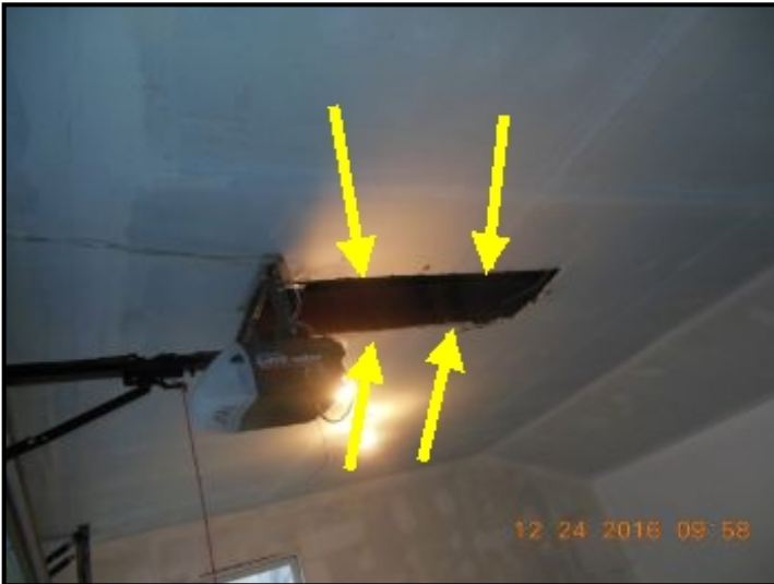
Open hole noted at access to garage attic space
