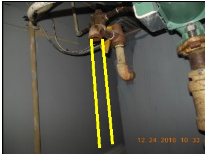
Missing TPR extension pipe noted on boiler
