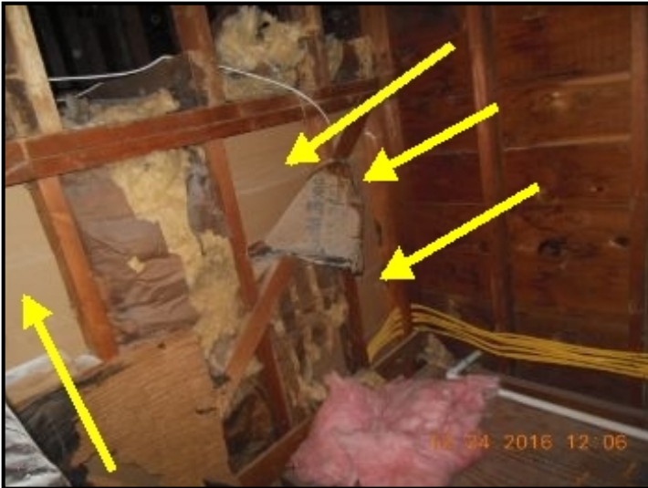
Missing insulation noted on vertical walls in attic
