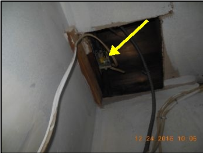
Open junction box noted in garage attic space
