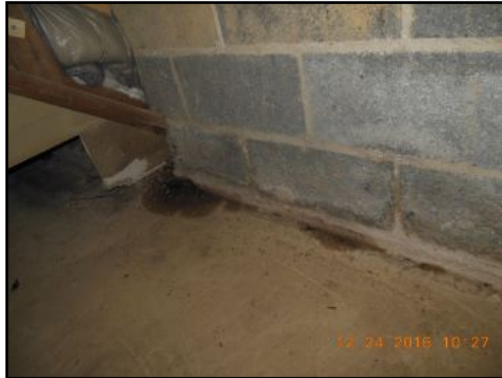
Moisture seepage up from floor noted near stairs in crawlspace
