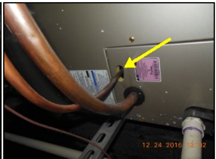
Wide open hole noted at evaporator coil area
