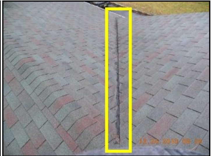
Roof cement repairs noted in one valley
