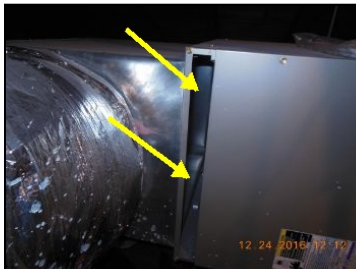
Missing filter noted at air handler in attic
