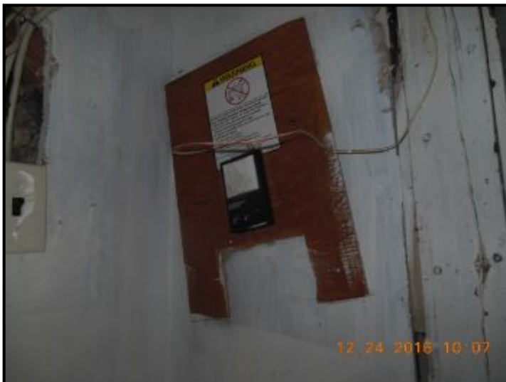
Plywood behind garage vehicle door push button is loose on wall
