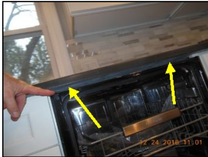
Dishwasher is not secured in place
