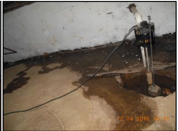
Wet floor around sump pit indicates water drainage system is inadequate
