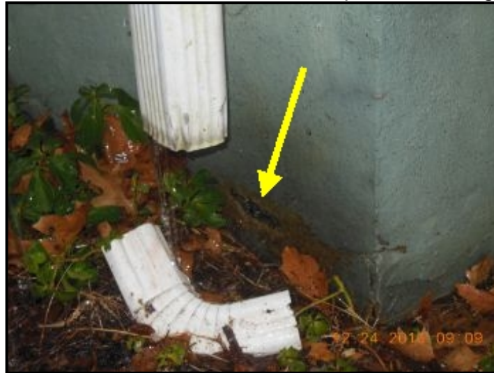
Minor erosion damage was noted on foundation wall from improper downspout drainage
