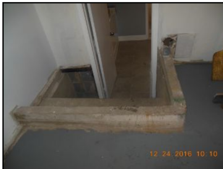
Missing handrail at stairwell in garage
