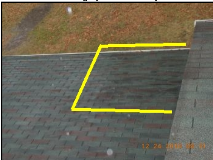
Heavily weathered curling shingles noted on rear roof of garage
