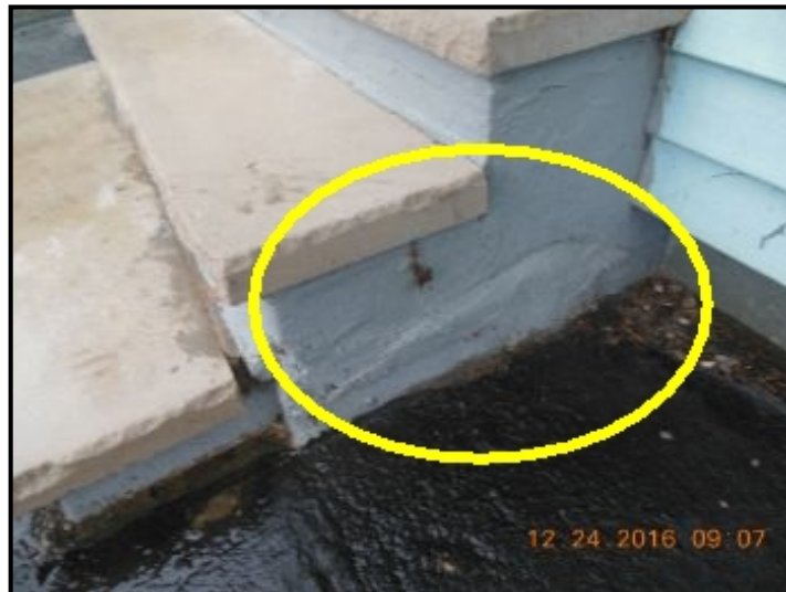
Swollen concrete stucco noted on side of porch indicating damage
