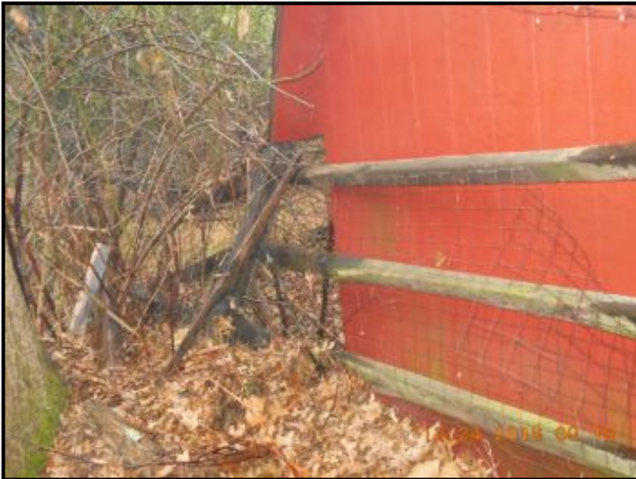
Extensive damage noted to fence around pool
