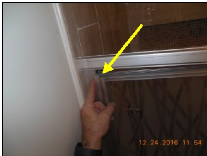
Shower door is improperly installed and loose at bedroom bathroom
