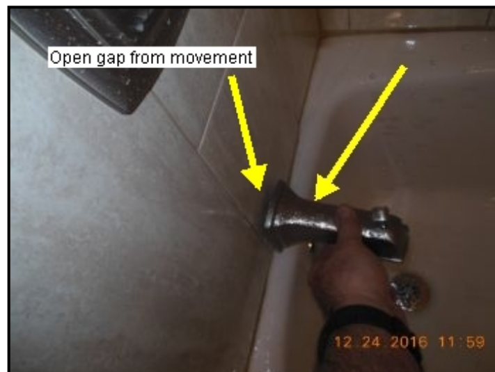
Tub faucet moves significantly in wall at upper level hallway bathroom
