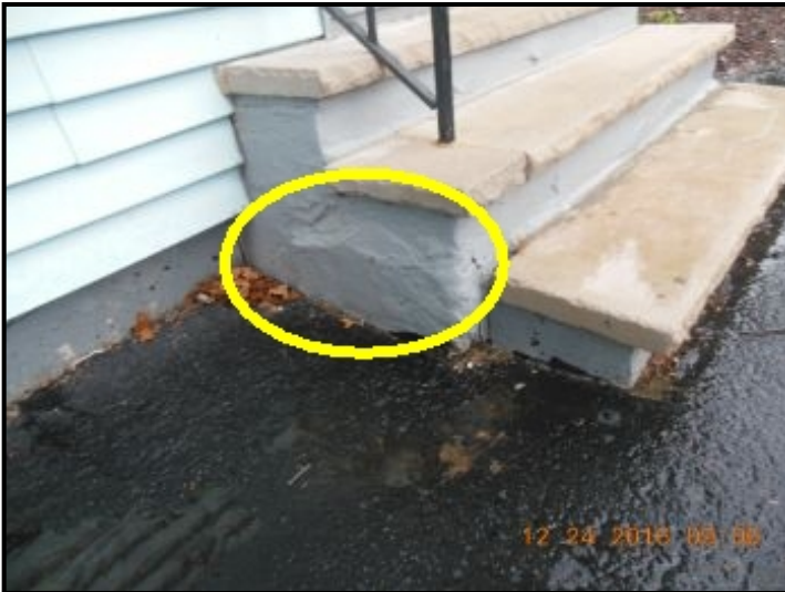
Swollen concrete stucco indicating damage to blocks under stucco
