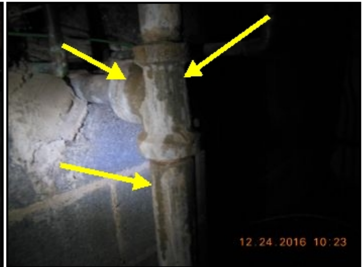
Wet stains on pipes indicate active leakage
