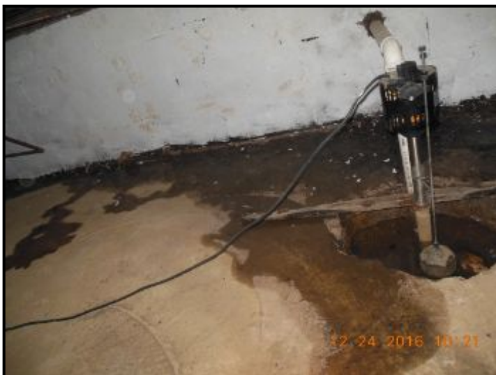
Wet floor in crawlspace indicates sump pits and pumps is inadequate in crawlspace
