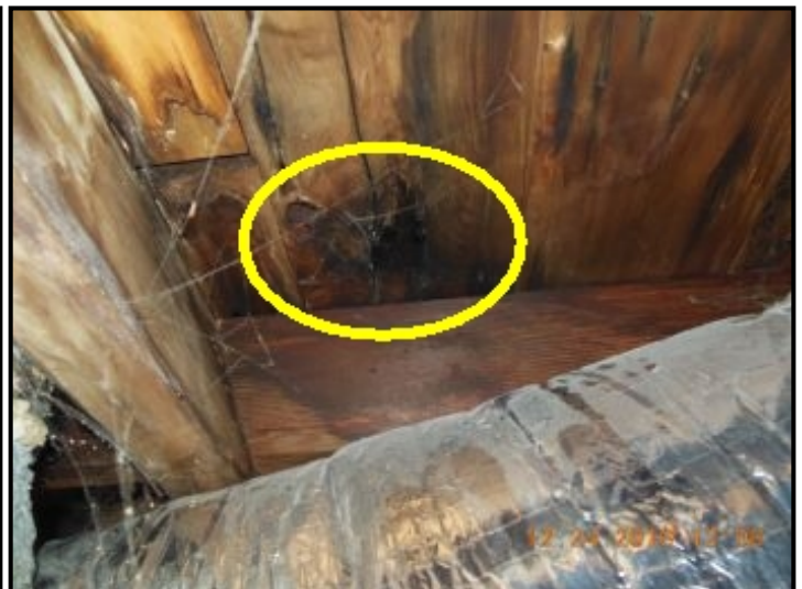
Active leak noted in roof by wet wood and dripping water
