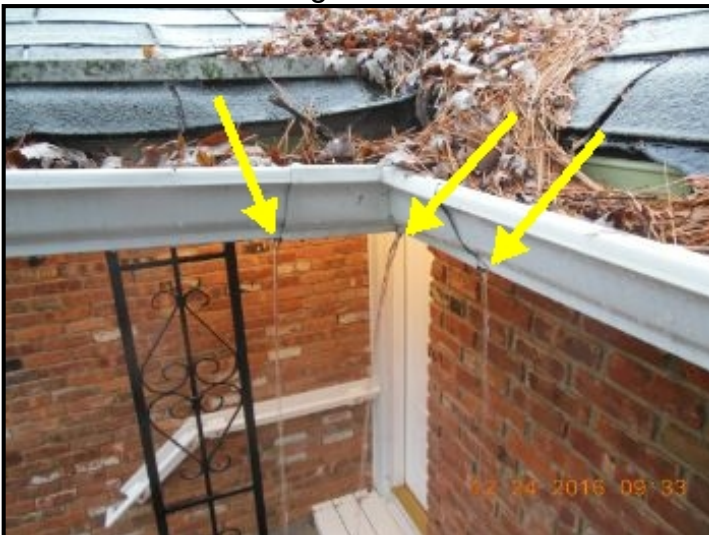
Gutters are leaking at seams
