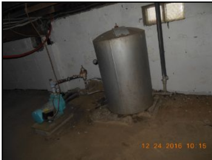
An above ground well pump is installed in the crawlspace
