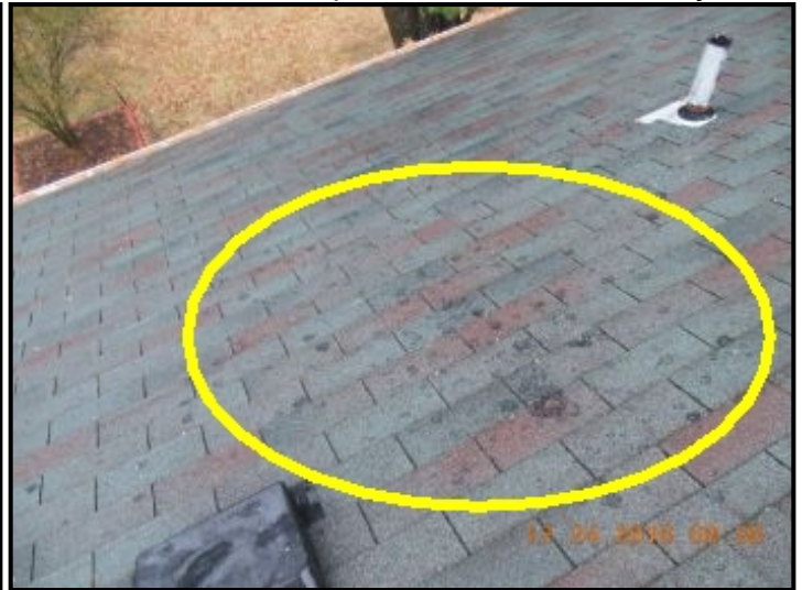
Some worn damaged batches of shingles on rear roof
