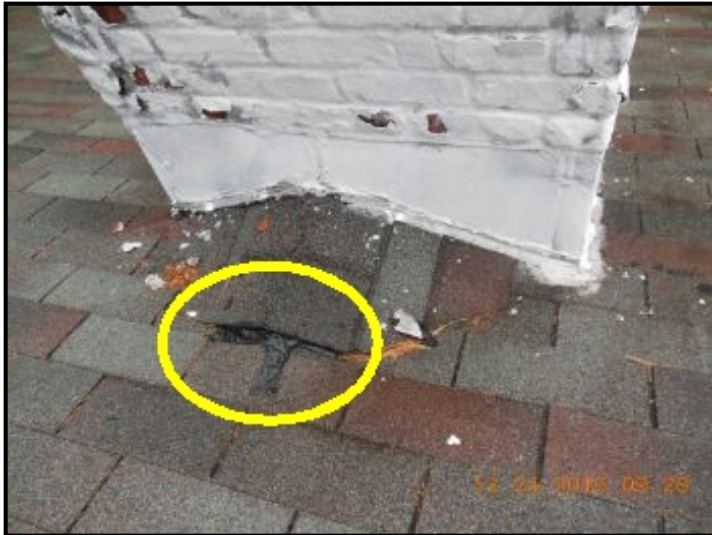
Roof cement repairs noted
