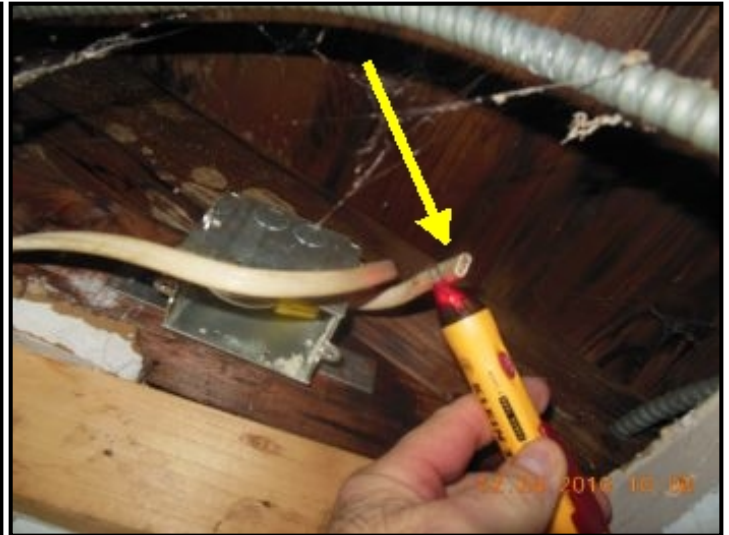
Cut live wire noted hanging above garage ceiling from open junction box
