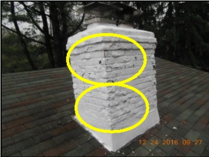
Spalling damage noted to mainy bricks on fireplace chimney
