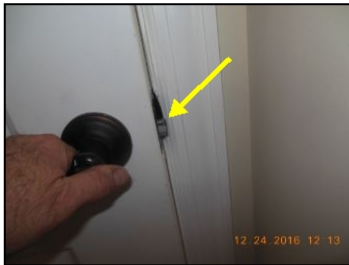
Upper level bathroom entry door does not latch shut
