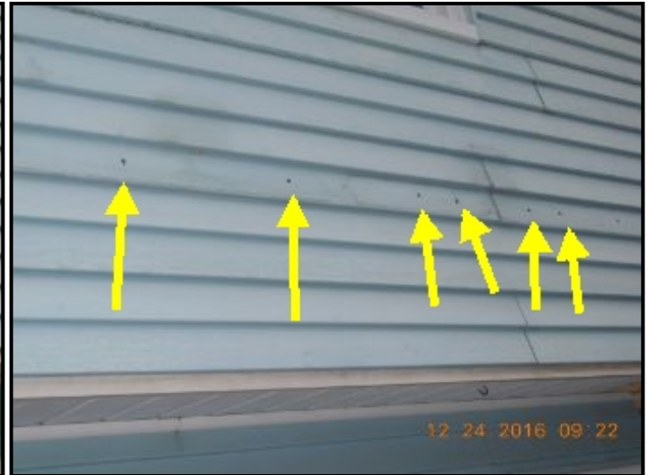
Open holes were noted in vinyl siding from removed deck awning cover
