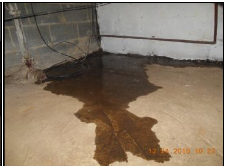
Wet floor in crawlspace indicates sump pits and pumps is inadequate in crawlspace
