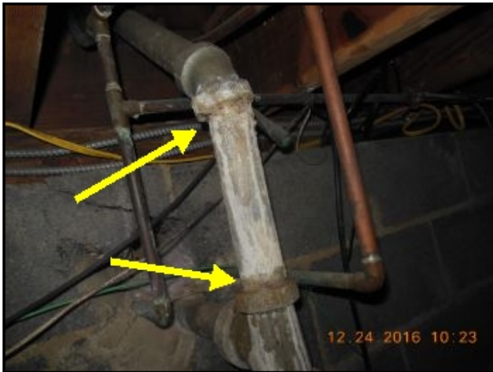
Corroded patched and leaking waste drain pipe in crawlspace
