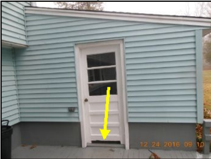
Bottom of service door is missing
