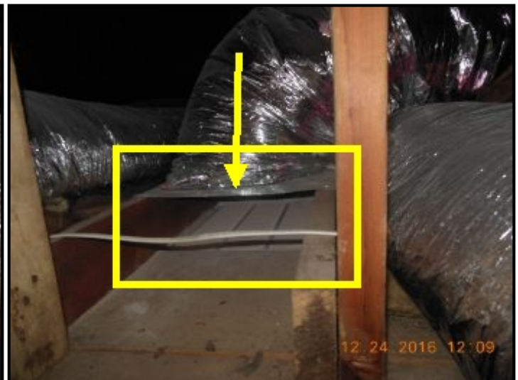
Another angle showing wide open holes between return duct flange and ceiling
