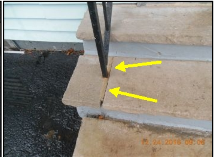
Open cracks in mortar joints on concrete steps
