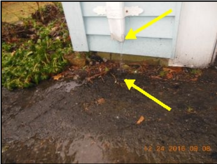
Water is draining next to foundation blocks
