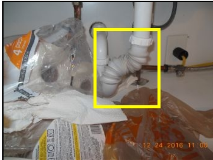
Improper ribbed drain pipe is installed under kitchen sink
