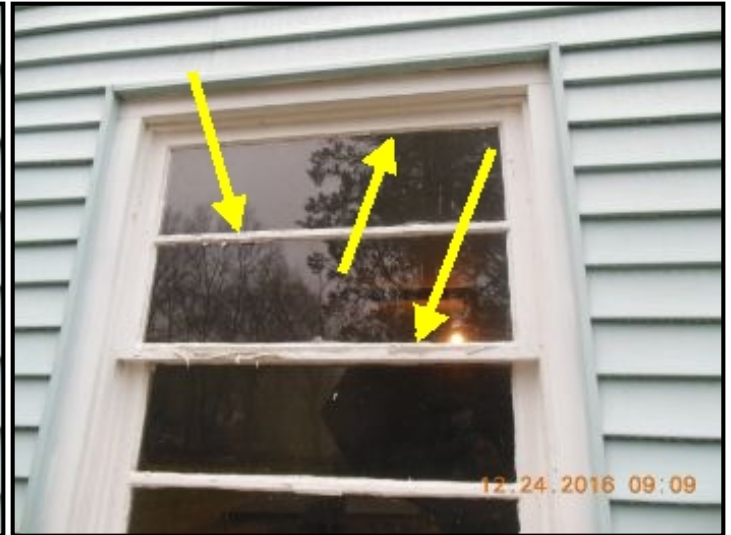
Peeling paint and missing putty noted on window glass
