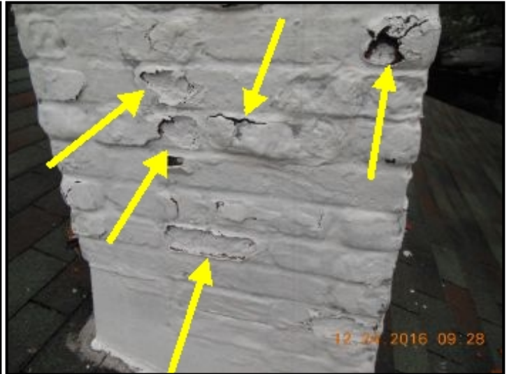
Closer look at brick damage on fireplace chimney
