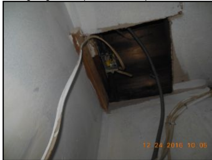
Open hole noted in garage firewall ceiling
