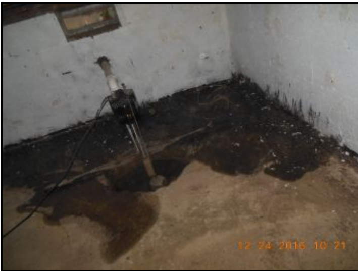
Wet floor noted in crawlspace indicating water drainage system is inadequate for water control
