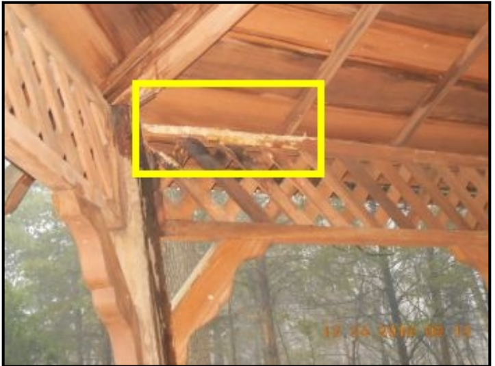
Rodent damage noted to gazebo structure under roof
