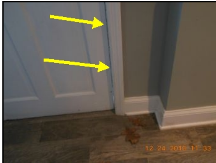
Open gaps at side of rear entry door
