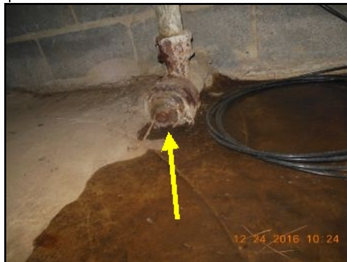
Corroded and leaking galvanized drain line at clean out cap
