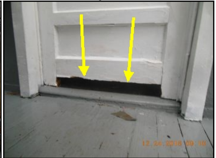
Closer look at damage to bottom of service door
