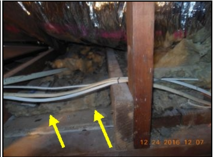
Old insulation in attic is batted down and thin
