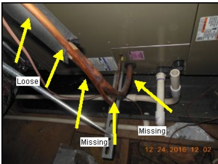
Loose and missing insulation noted on refrigerant line in attic
